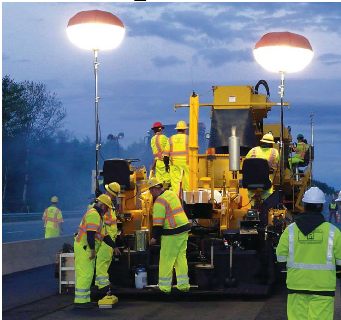
▲ Night Moves. Pike Industries Inc. paving crew working on a New Hampshire ARRA-funded highway job; the state mobilized quickly to get projects ready.
